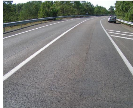
Figure C9 Poor transversal joint
