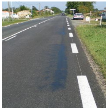
Figure C10 bleeding or fattening up of UTLAC (loss of macro-texture)
