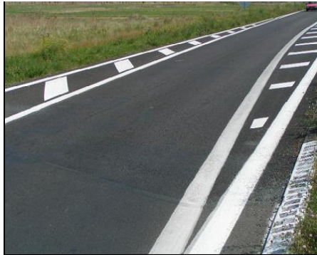
Figure C8 Transverse bump and localised fretting
