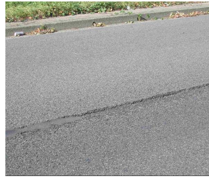
Figure C7 Ravelling on longitudinal joint
