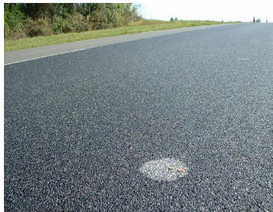
Figure C4 Satisfactory UTLAC – homogeneous texture
